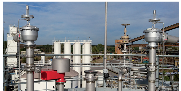
Cryogenic Storage Tank
