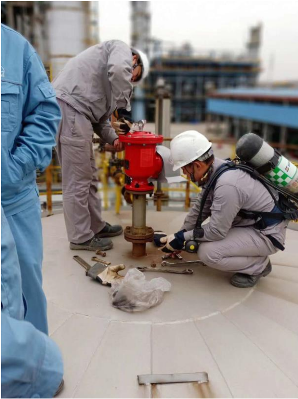
Picture 2: The PROTEGO® valve was installed
