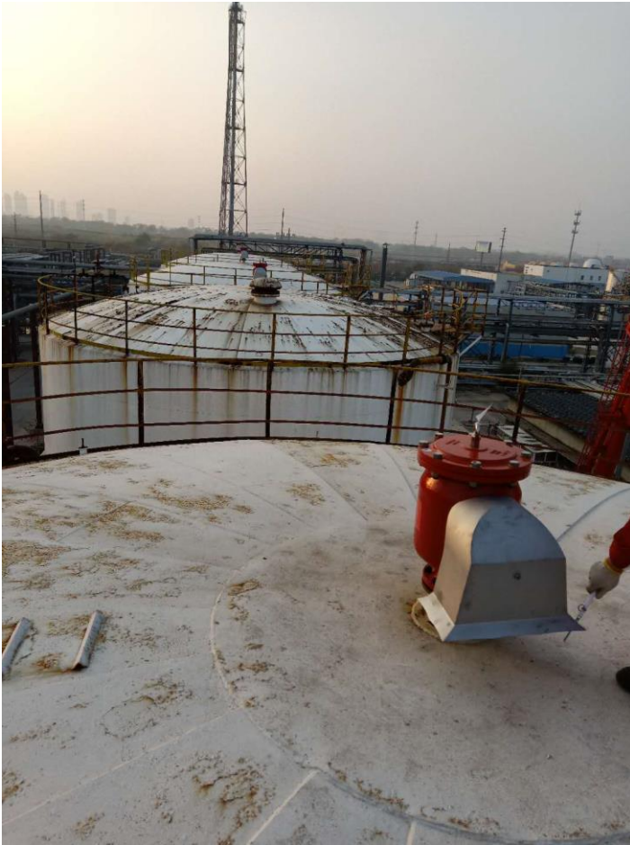
Picture 4: All of the tanks are protected by PROTEGO® valves
